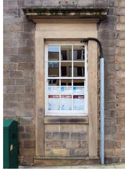
Altered door and intrusive cable trunking
