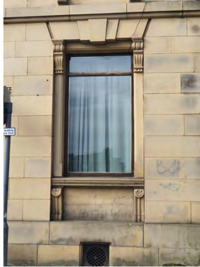
Inappropriate window design
