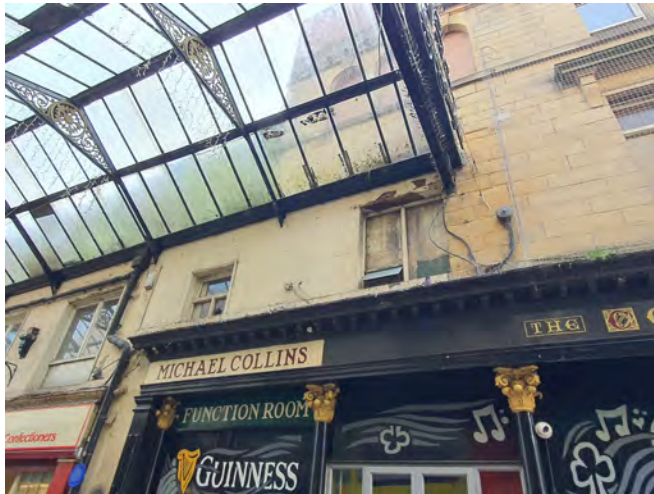
Guano accumulation, bird netting, bird spikes and poor maintained upper storey in the arcade
