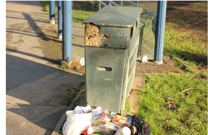
Rubbish bin in poor condition
