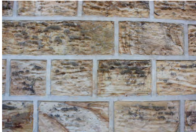
Strap pointing is not traditional and is inappropriate within the Conservation Area. Additionally, the use of cement mortar will cause further decay to the already weathered stonework
