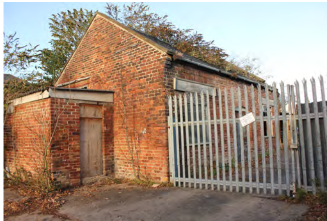
Canal Basin brick structure in poor condition, thought to have been formerly associated with the railway
