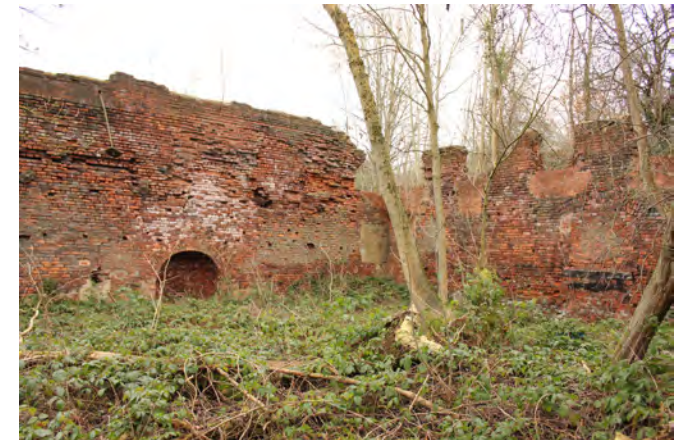
The Blowing Engine House (part of the Elsecar Ironworks and now within a Scheduled Area) is inaccessible and in poor condition
