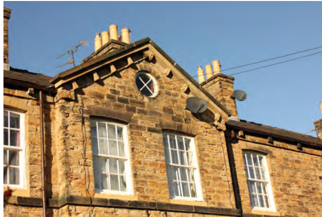
Satellite dishes, aerials and telephone wires attached to a listed building. Note that listed building consent is required
