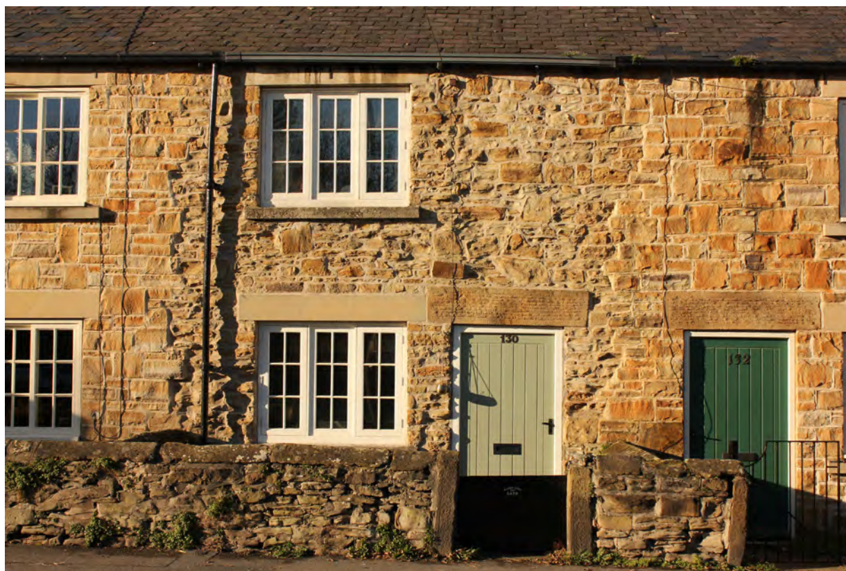
Different repair methodologies and on Reform Row have impacted on the uniformity of the façade
