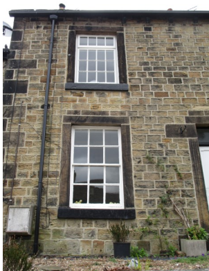
Plate 29: 6 over 6 sash window (bottom) on No. 12 Darton Road. The top window has been replaced
