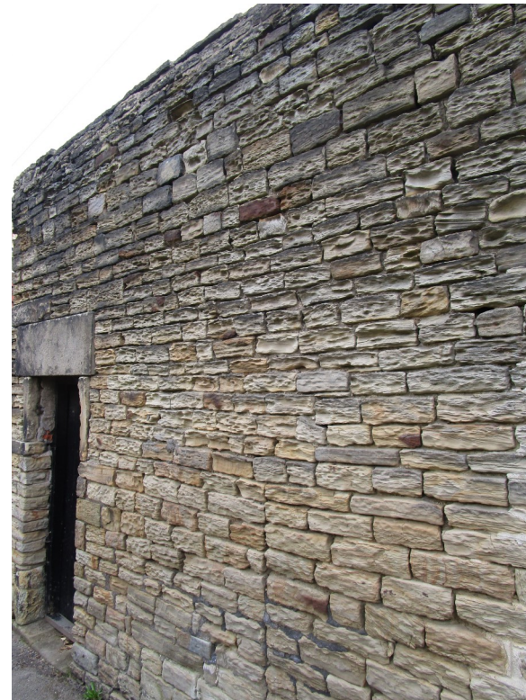
Plate 24: Sandstone outbuildings, rear of Victoria Cottage Institute, Darton Road - where cement pointing has been used in the past, the face of the stonework has eroded
