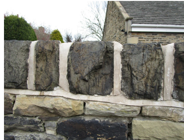
Plate 51: Ribbon and cement pointing detract from historic walling and is a cause of erosion
